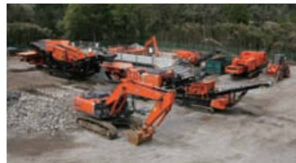
Hi-OSS demonstration site
